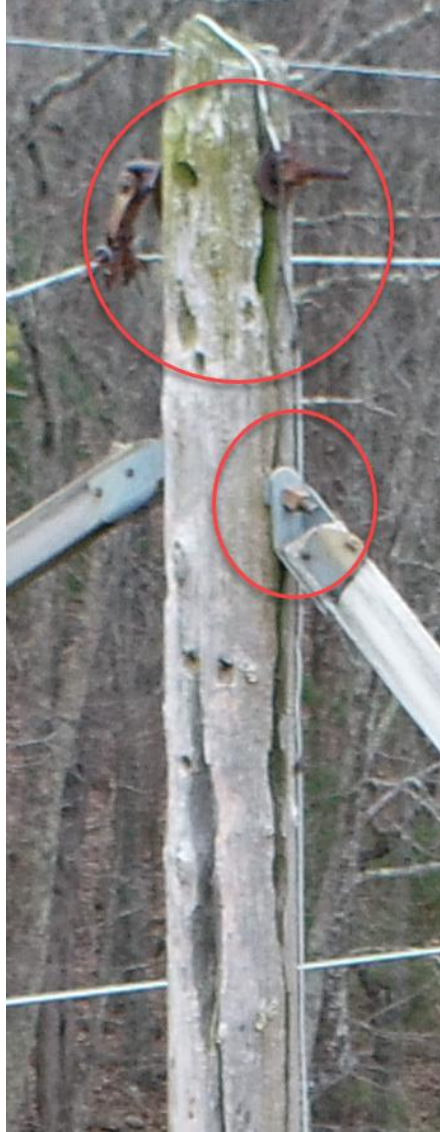
Figure 19: Component 3: Claytor – Fieldale 138-kV Line Structure 30-129: Several Large Pole Cavities and Severe Vertical Pole Splitting with Potentially Compromised Knee Brace and Shield Wire Attachment Points
