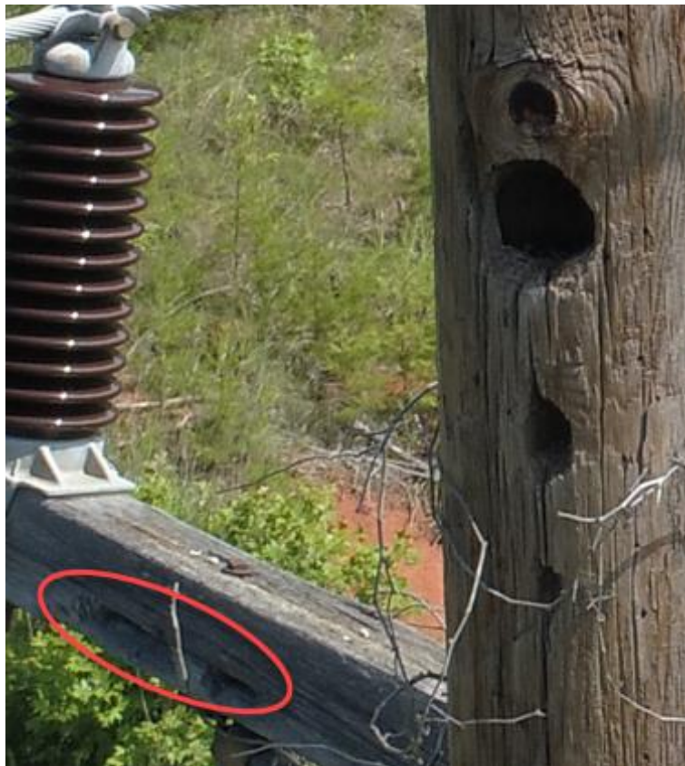
Figure 34: Component 3: Fieldale - Stuart 69-kV Line Structure 484-286: Multiple Woodpecker Holes and Crossarm Splitting
