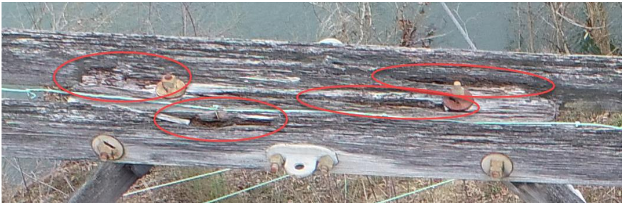
Figure 26: Component 3: Claytor – Fieldale 138-kV Line Structure 30-264: Crossarm Splitting and Decay
