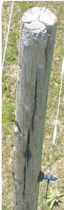
Figure 31: Component 3: Fieldale - Stuart 69-kV Line Structure 484-202: Upper Pole Splitting and Decay
