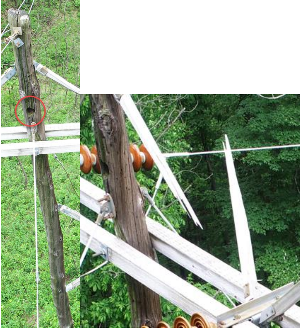
Figures 11 and 12: Component 2: Floyd – Stuart 69-kV Line Structure 452-45: Large Pole Cavity, Pole Decay, and Broken Knee Brace
