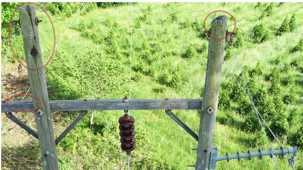
Figure 15: Component 2: Floyd – Stuart 69-kV Line Structure 452-76: Remediated Crossarm Failure, Crossarm and Pole Splitting, Pole Rot Top, and a Large Woodpecker Hole
