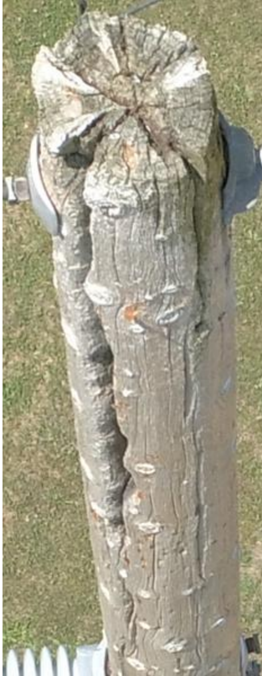
Figure 27: Component 3: Fieldale - Stuart 69-kV Line Structure 484-45: Severe Pole Splitting with Upper Pole Decay
