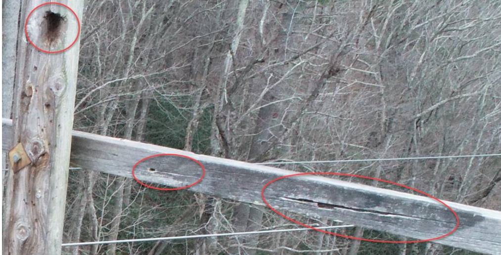
Figure 22: Component 3: Claytor – Fieldale 138-kV Line Structure 30-185: Crossarm Splitting and Decay and a Pole Cavity
