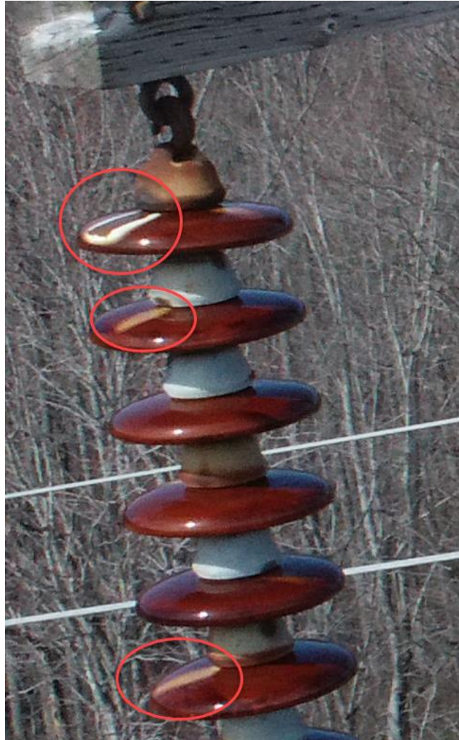
Figure 21: Component 3: Claytor – Fieldale 138-kV Line Structure 30-162: Multiple Flashover/Arcing Damage Indications to Insulator
