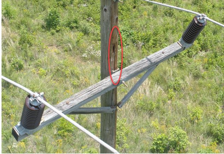
Figure 28: Component 3: Fieldale - Stuart 69-kV Line Structure 484-76: Severe Pole Splitting at Crossarm Attachment with Slight Crossarm Rolling
