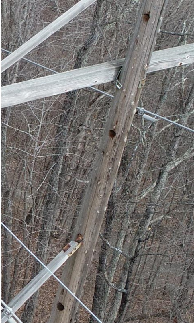
Figure 25: Component 3: Claytor – Fieldale 138-kV Line Structure 30-230: Several Large Woodpecker Holes
