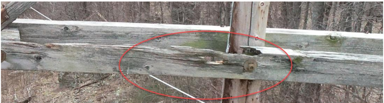
Figure 20: Component 3: Claytor – Fieldale 138-kV Line Structure 30-148: Severe Crossarm Splitting at Pole Attachment Point
