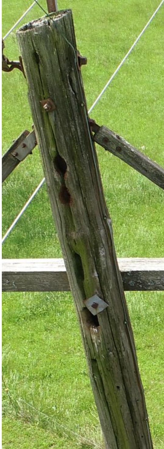
Figure 10: Component 2: Floyd – Stuart 69-kV Line Structure 452-20: Severe Pole Splitting, Decay, and Woodpecker Holes
