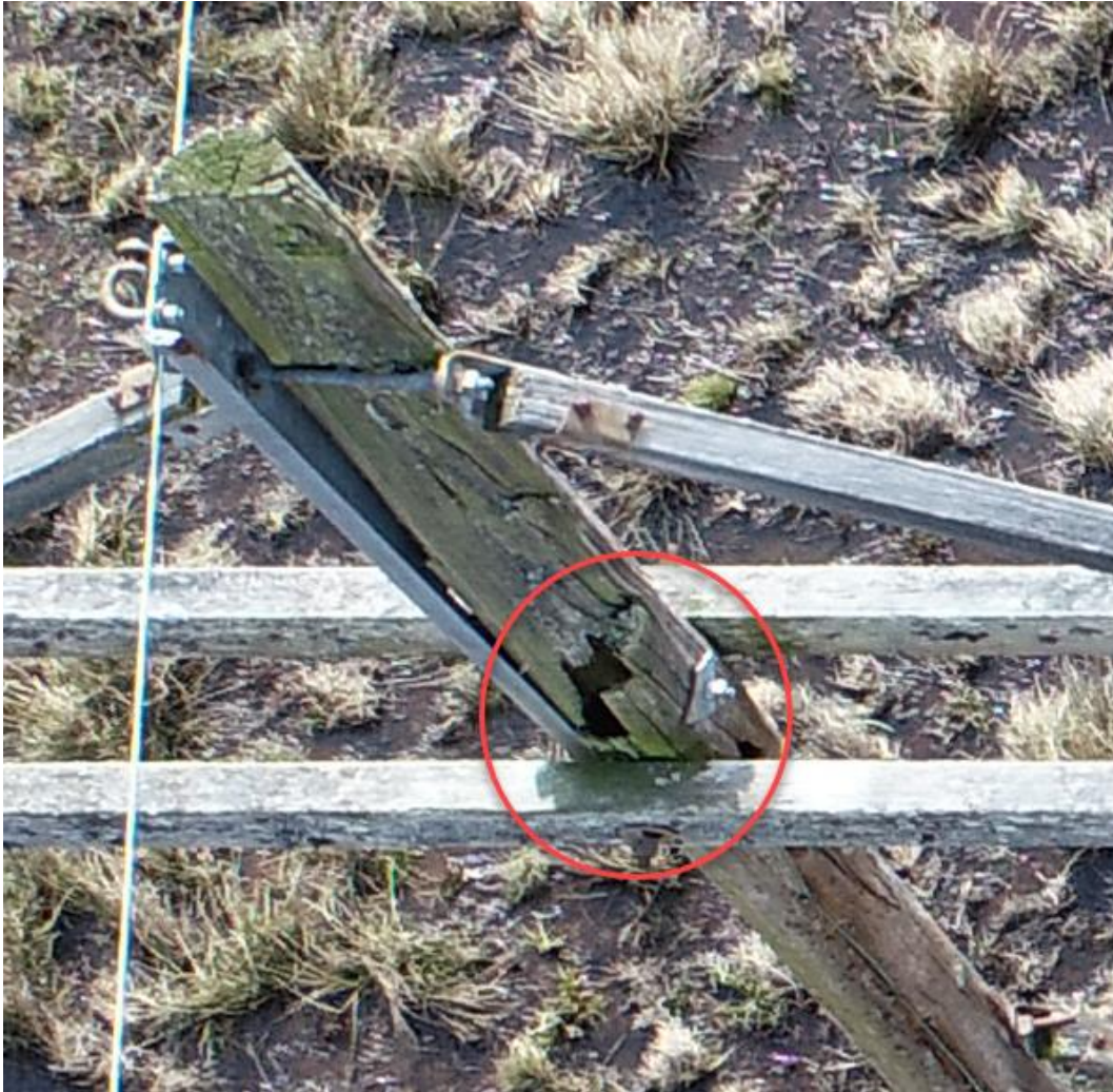
Figure 18: Component 3: Claytor – Fieldale 138-kV Line Structure 30-114: Severe Upper Pole Splitting Impacting Structural Integrity at Crossarm Attachment Point
