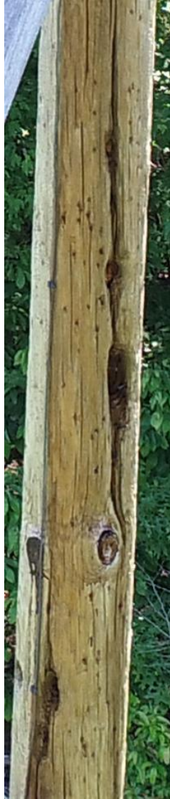
Figure 16: Component 2: Floyd – Stuart 69-kV Line Structure 452-100: Pole Splitting and Cavities
